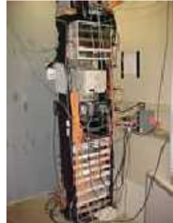
Figure 5: the wiring hub
